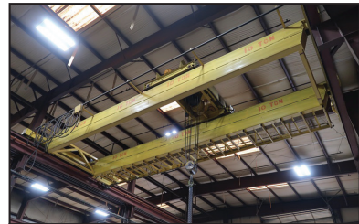
(2) 10-TON BRIDGE CRANES
