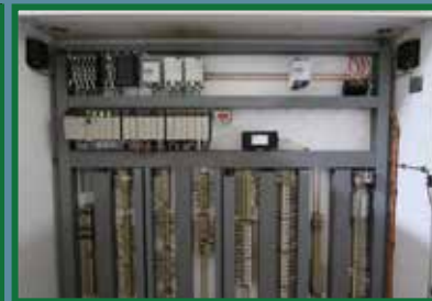
2020 ALLEN BRADLEY LOGIX 5561
