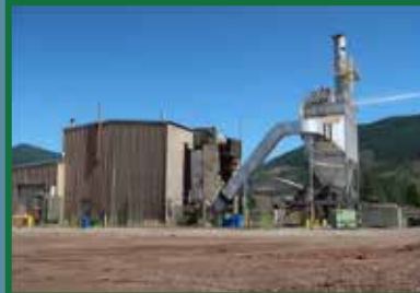
2018 REBUILT ELECTRO STATIC
