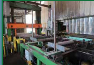
MANUAL BANDING STATION W/LUMBER SQUEEZE
