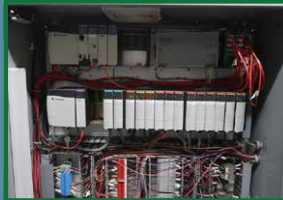
2020 ALLEN BRADLEY LOGIX 5572
