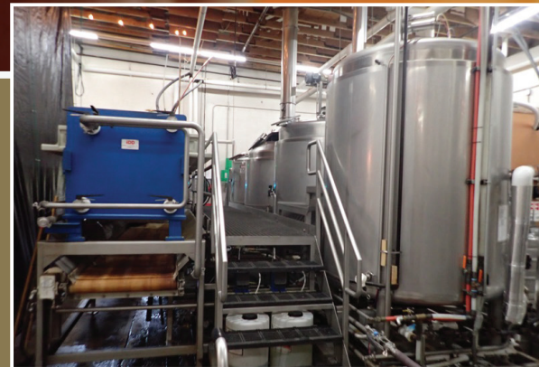
IDD 20HL 4-VESSEL HIGH EFFICIENCY BREWHOUSE
