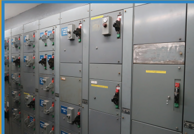
ALLEN BRADLEY CENTERLINE 2100
