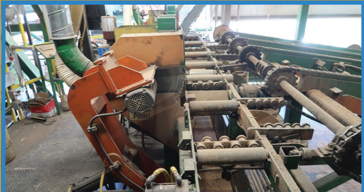
HULA SAW TIMBER CUT OFF STATION
