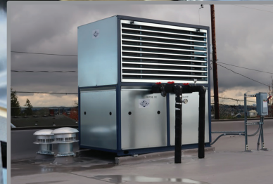
PRO REFRIGERATION CHILL STAR
