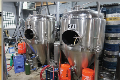
(2) 6BBL S/S JACKETED FERMENTATION TANKS
