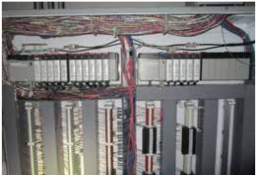
ALLEN BRADLEY PLC'S
