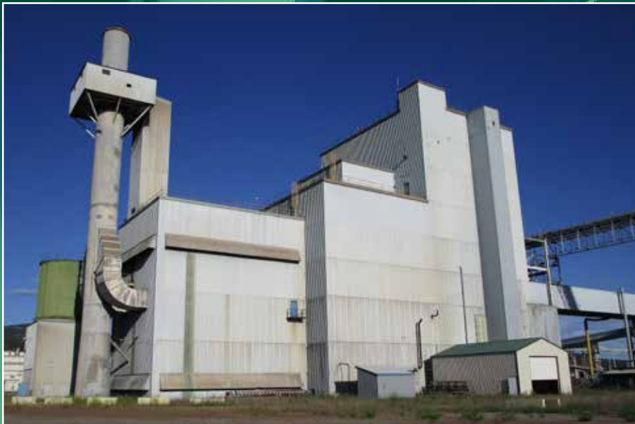
1980 COMBUSTION ENGINEERING TYPE VU-40 MULTI-FUEL BOILER
