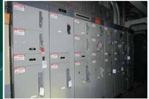
(60±) SECTIONS OF ALLEN BRADLEY CENTERLINE MCC'S
