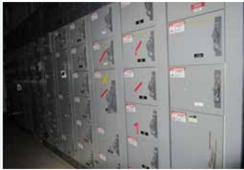
(60±) SECTIONS OF ALLEN BRADLEY CENTERLINE MCC'S
