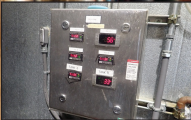
6-VESSEL TEMP CONTROL PANEL
