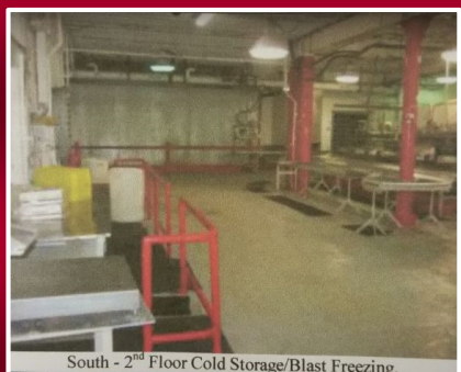
South - 2 nd Floor Cold Storage/Blast Freezing.
