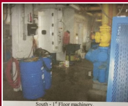
South - 1 st Floor machinery.
